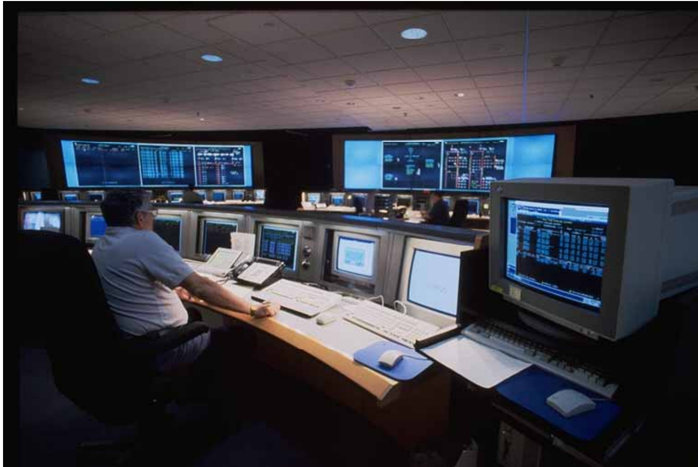
Xcel Energy Control Room Minneapolis
