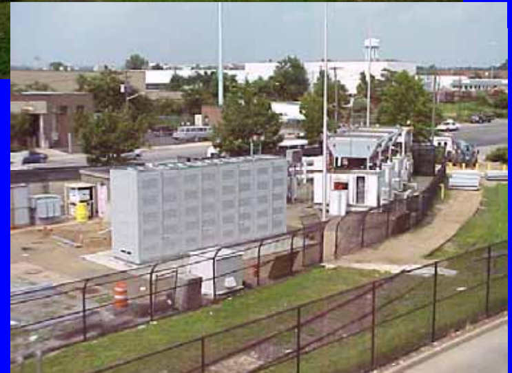
Three 600-HP compressors + 1 MW NaS battery
