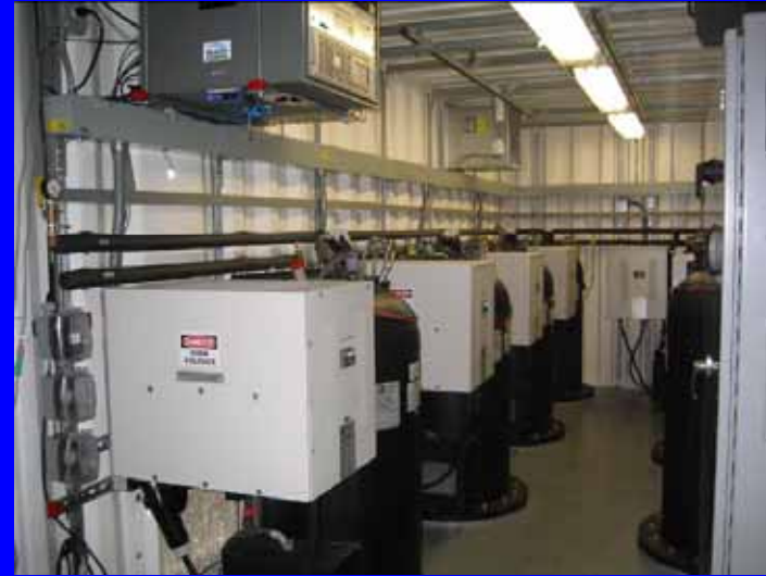
Containerized 7 Flywheel System
