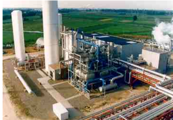
1,800 MTPD Air Separation Plant
